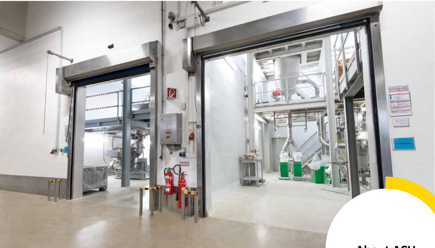
Separately enclosed production facilities for your product safety
